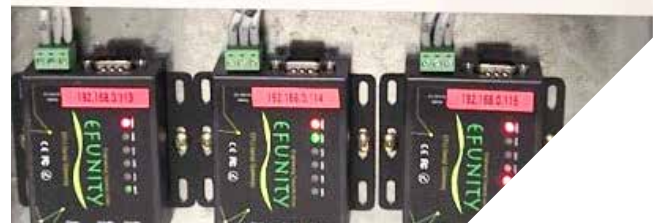
Installed sub-sensors to enable a more precise monitoring of energy consumption at SETSCO's premise.
